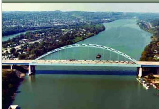
Practically, the span-to-rise ratio for a tied arch can vary between 4 and 7. Often, a more pleasing appearance is realized in the 5.5 to 6 range.
